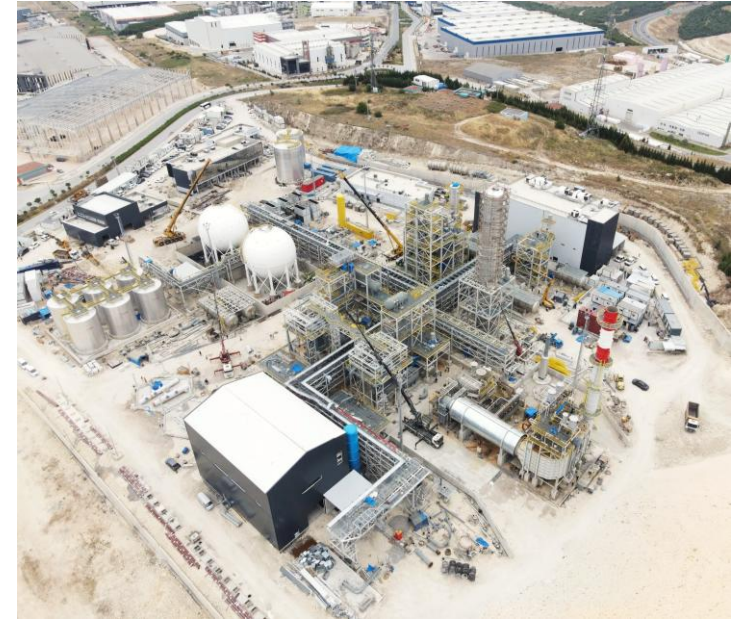
Integrated plant view
