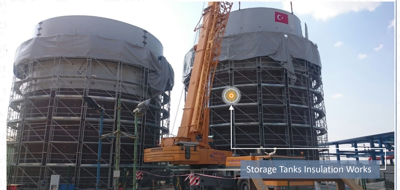
Hamitabat Demineralized Water Storage Tanks
