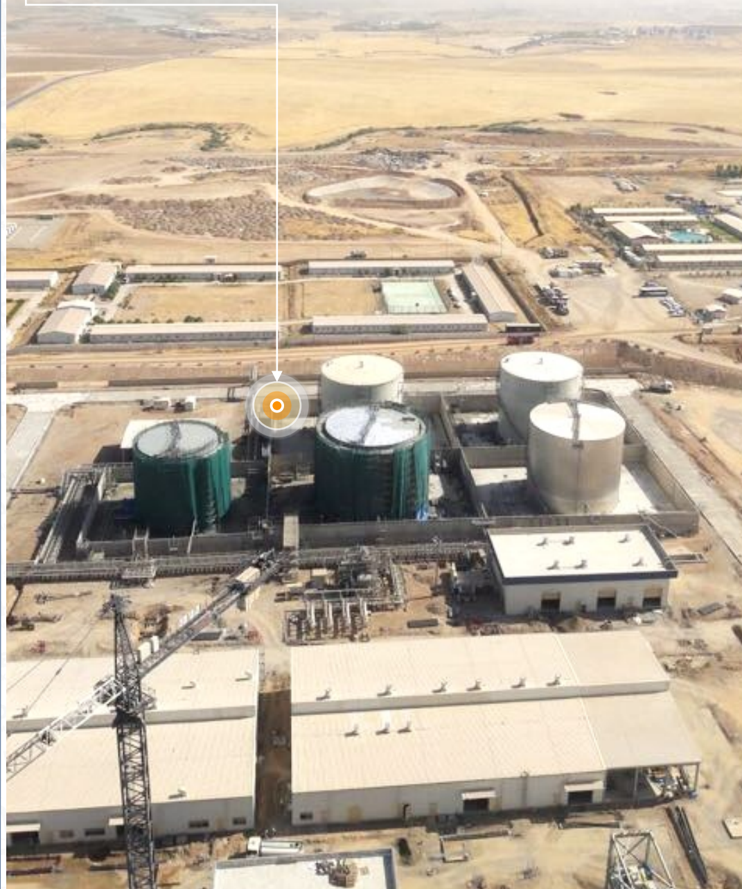
Fuel Oil and Diesel Storage Tank Farm
