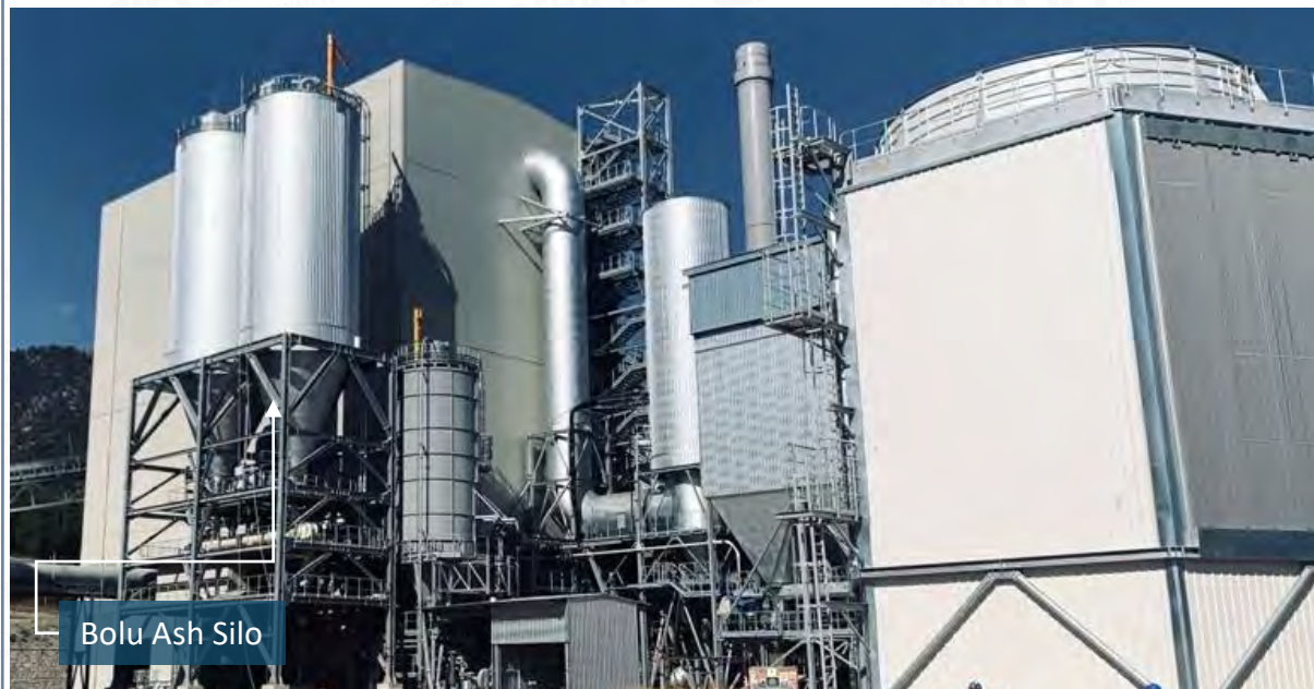
Bolu Biomass Plant Process Equipment
