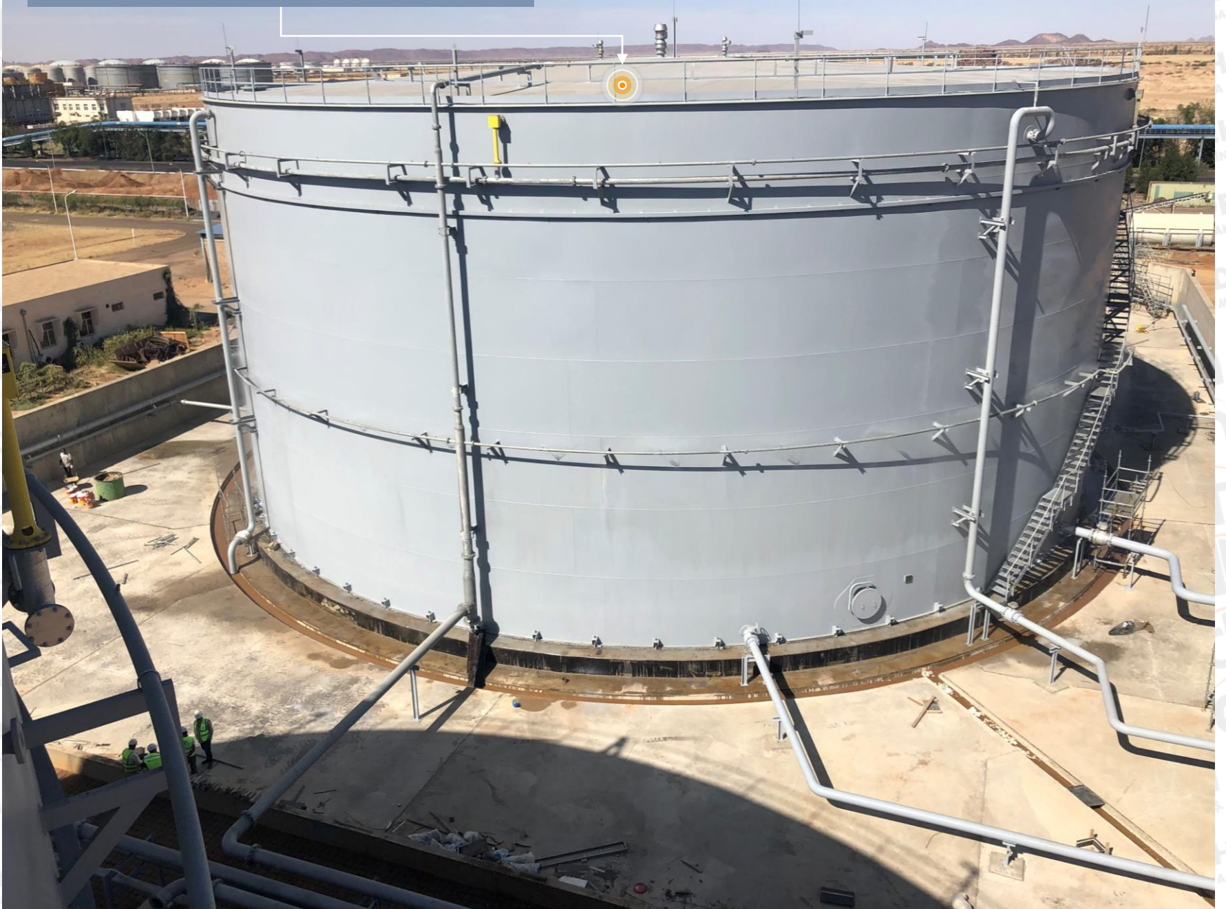
Garri 3 - 750 MW SCPP Heavy Fuel Oil Tank
